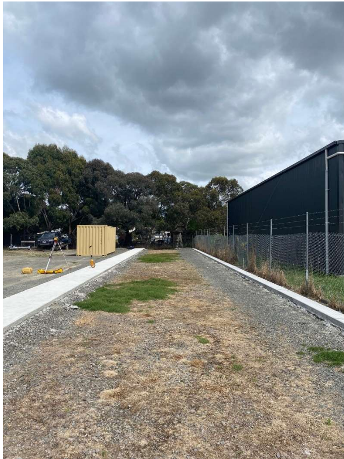
View Looking along North Titla boundary. Recently installed footings currently unused, natural surface graded to drainage line.
